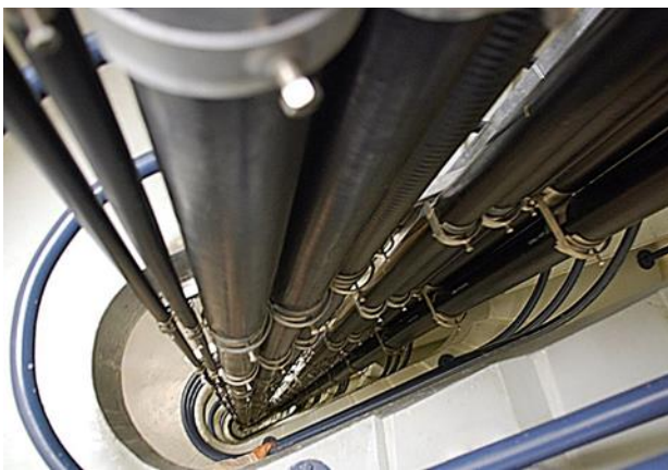
6. Rigid cable installed in a broadcast tower
